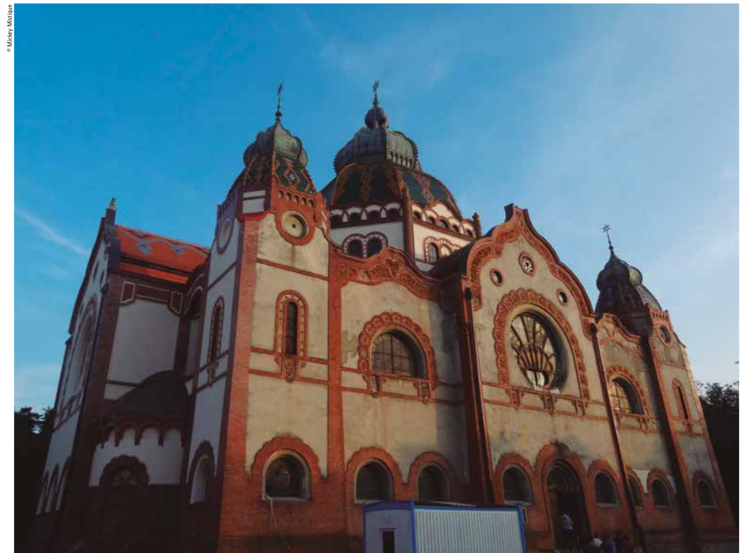
General view of the Synagogue before restoration was complete, with the roof tiling only partially replaced
