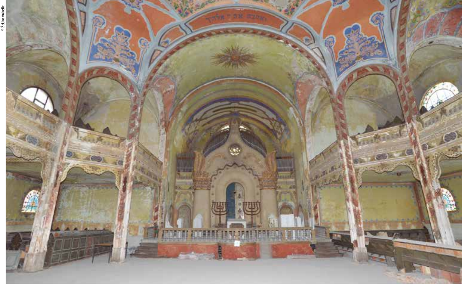
Decades of neglect and misuse had wrought its havoc on the interior. In the debate on whether to opt for minimal intervention or fully recover the original appearance, the latter finally prevailed
