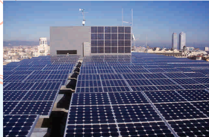
Photovoltaic solar panels of the City Hall
