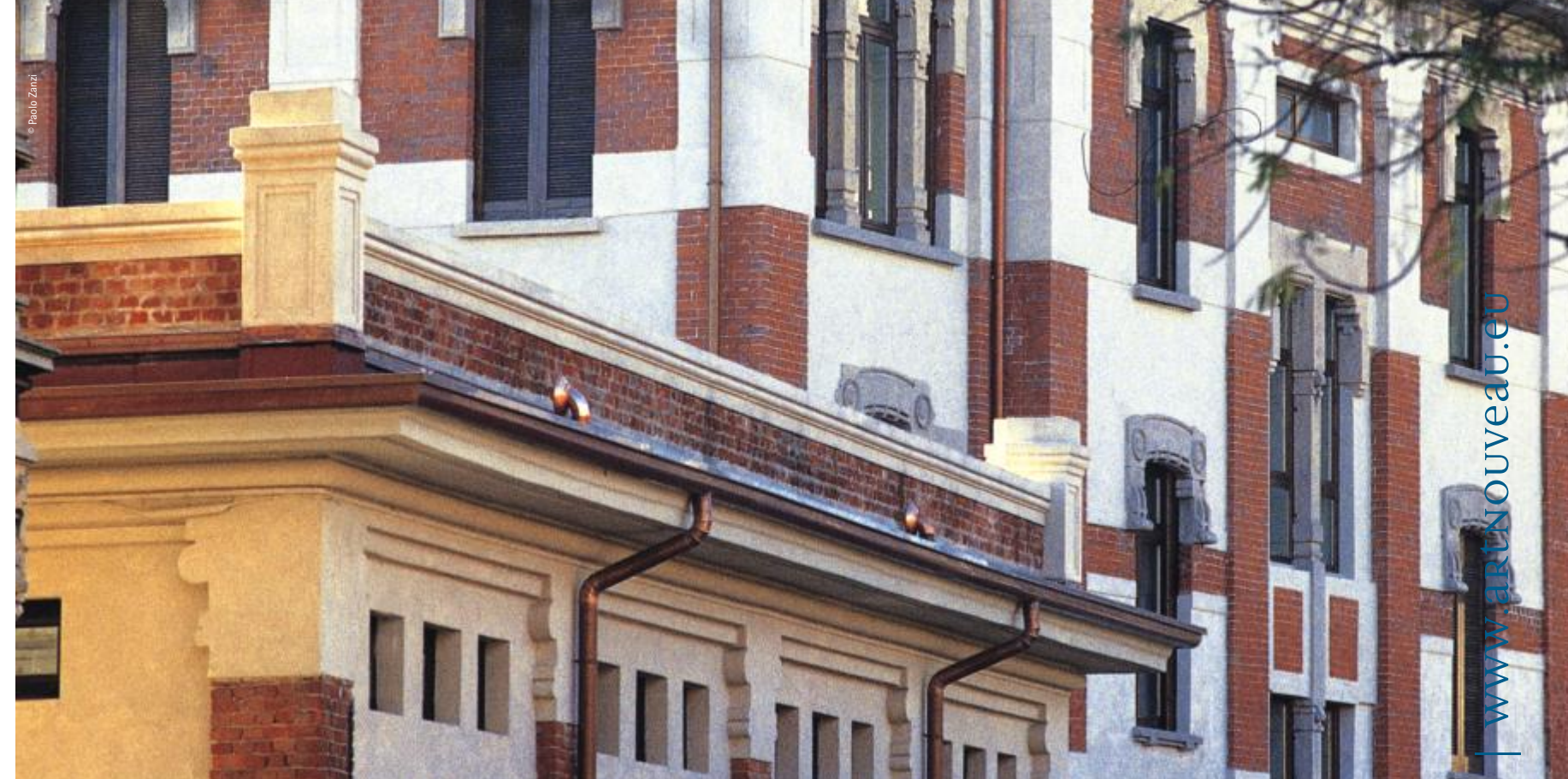
Molini Marzoli Massari. Tecnocity. Detail of the restored façade / Detall de la façana rehabilitada.
