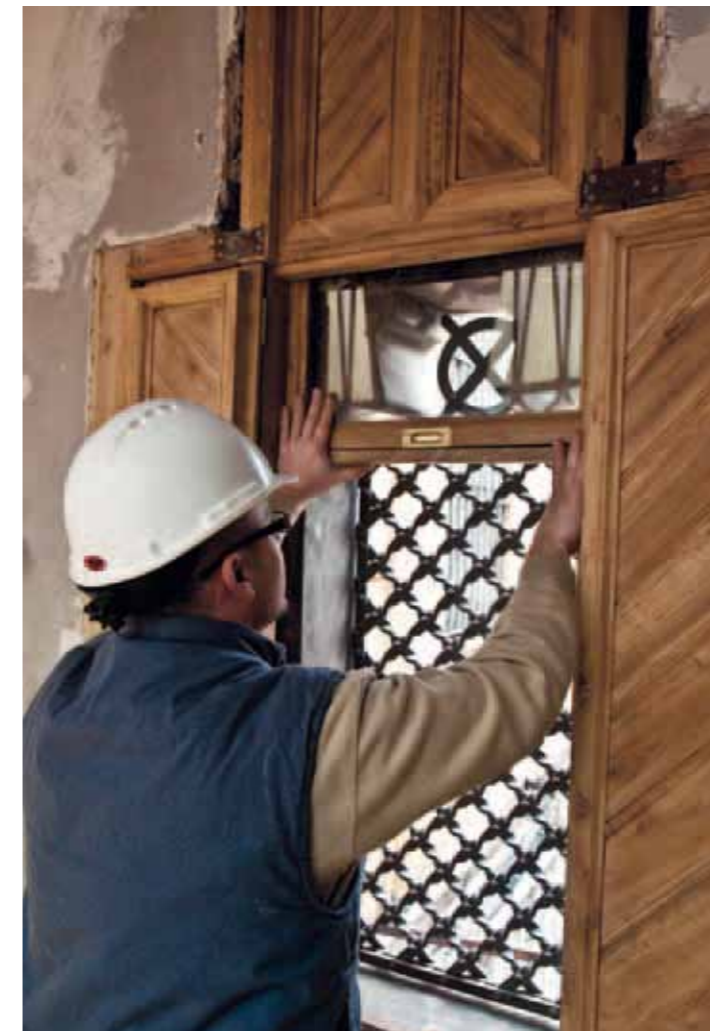
The windows were taken apart, restored and then put together again Els finestrals van ser desmuntats, restaurats i finalment recol·locats
